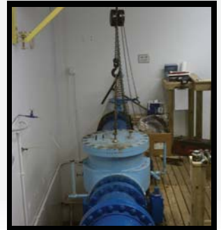
16" GA Valve in Glenwood, IL
